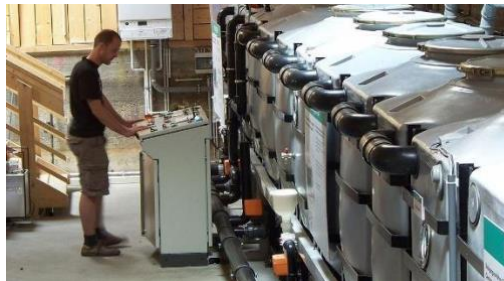
Greywater treatment plant at Water House, Berlin, Germany. Photo: Erwin Nolde.
